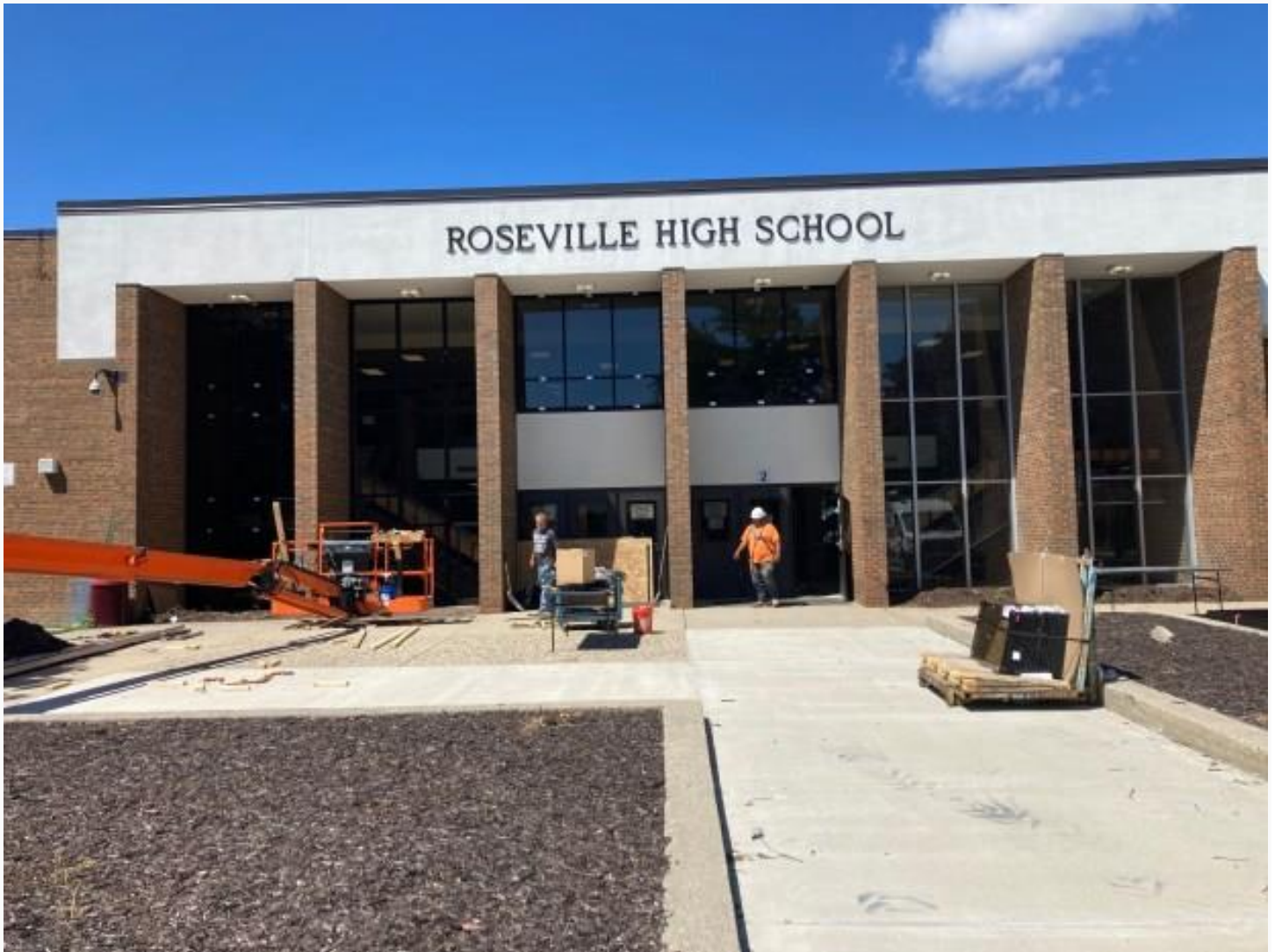
A crew works to install new safety glass at Roseville High School. (MITCH HOTTS — THE MACOMB DAILY)
